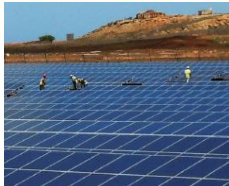
5 MW Solar PV, in Praia, Cape Verde Commissioned November 2, 2010
