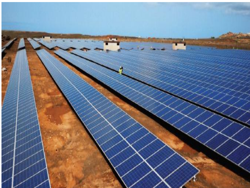
2.5 MW Solar PV, in Sal, Cape Verde Commissioned October 1, 2010
