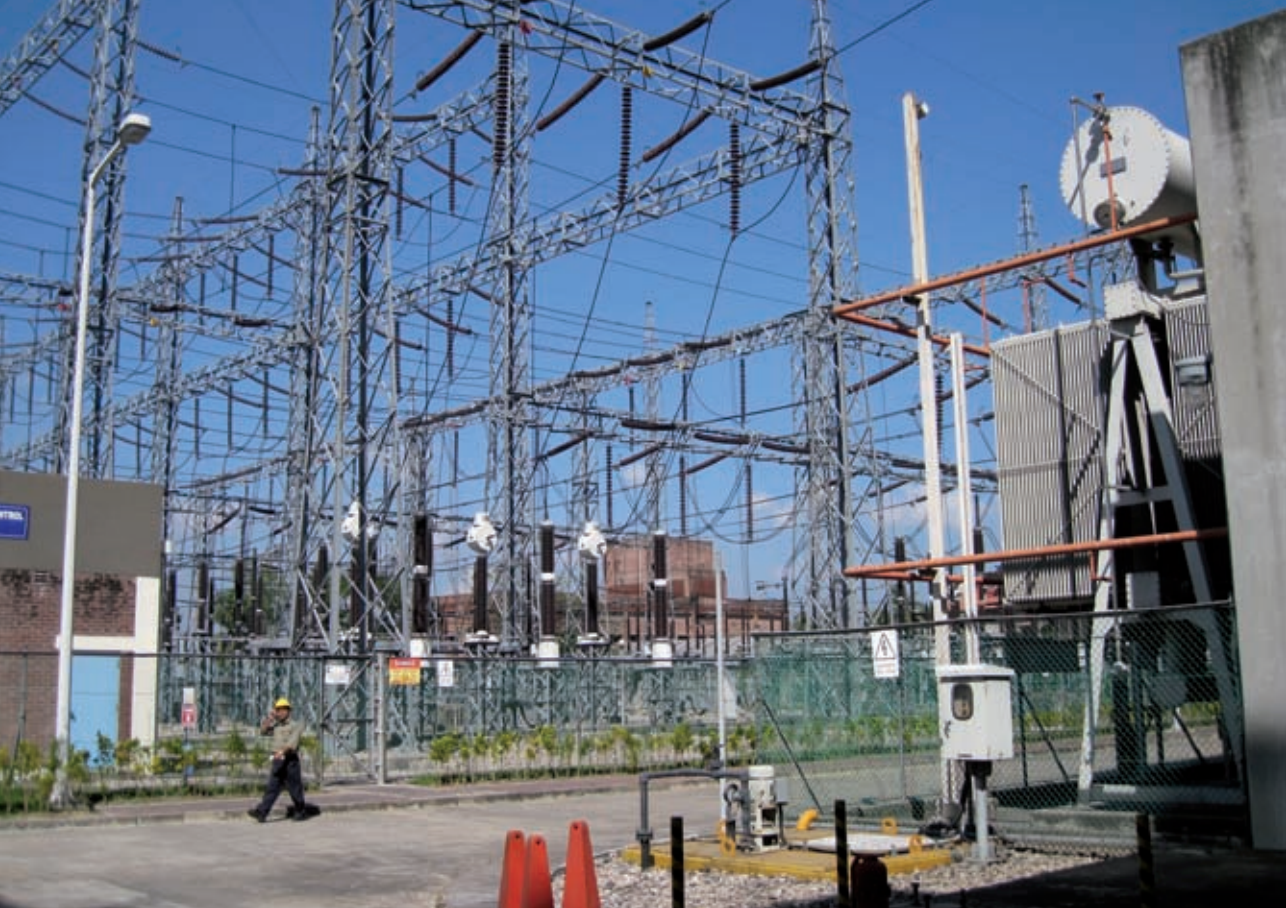
Haripur Power Plant in Dhaka (Bangladesh)
