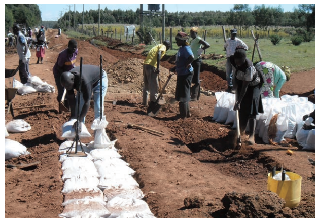
Community Road Empowerment (CORE) Sustainable Rural Road Maintenance using Do-nou Technology by the Community (Phase II) in Kenya
