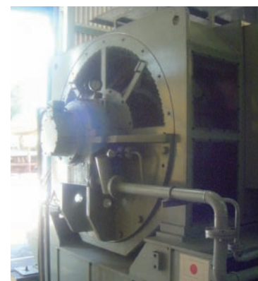
Installed Diesel Engine Generator (Lungga Power Station)
