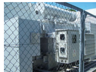
Transformer in Ranadi S/S (Ranadi Substation)
