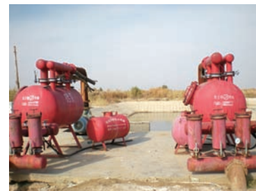
Pumping machine and fertilizer mixing machine (Tacheng)
