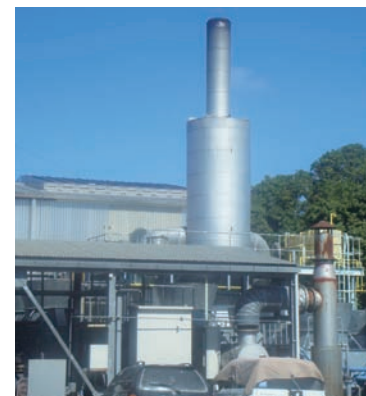
Exhaust Tower (Lungga Power Station)
