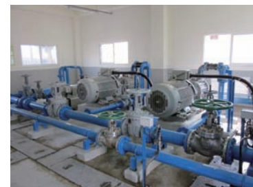
Adasiya pumping station
