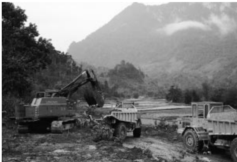
Construction of a forest road near Ham Yên, using heavy machinery from Sweden. Photo: Heldur Netocny/Phoenix
