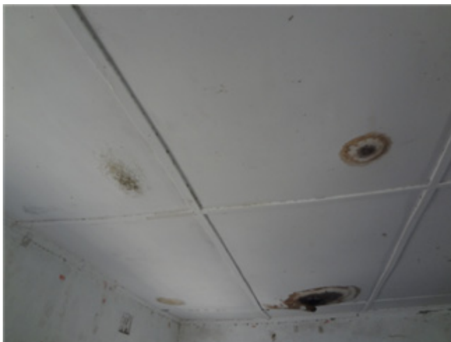
<Figure 3-5> Leakage on ceilings
