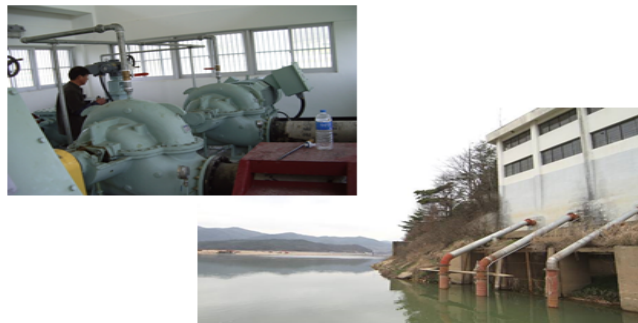
[Figure 10] Pumping Station - Reference Photos
