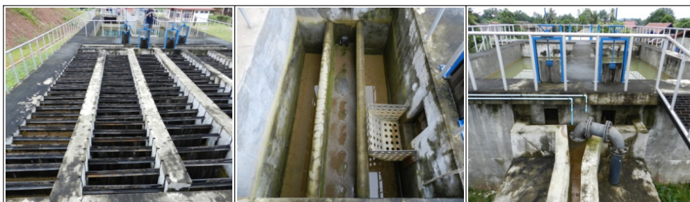
Photo 2-5 KOICA drinking water system (PMC: K-Water)
