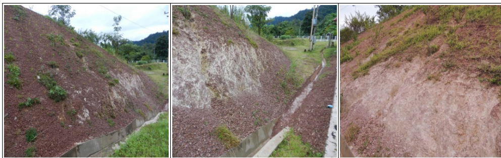
<Photo 4-1> Loss of slope soil due to lack of vegetation
