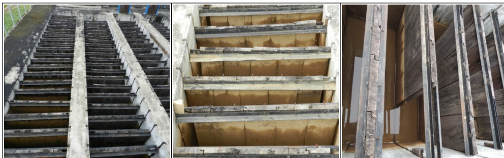
<Photo 4-3> Baffles chipped off and broken
