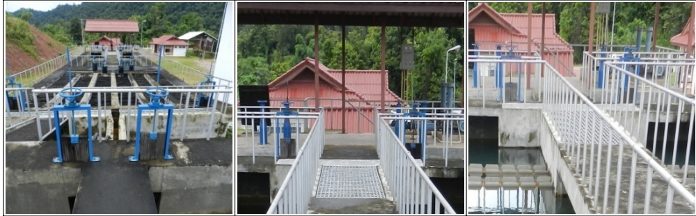
<Photo 4-4> No protection from potential pollutants due to passage
