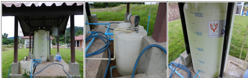
<Photo 4-2> Exposure of chlorine treatment facility to sunlight
