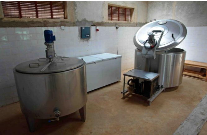
Figure A5 MMCS – new milk processing equipment awaiting final installation
